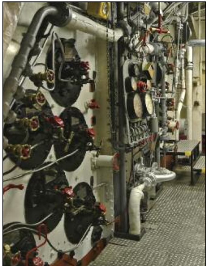
No. 2 Boiler Room
